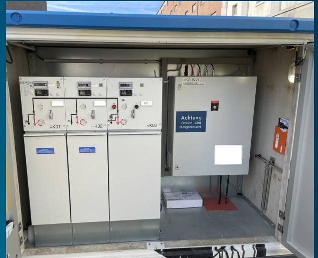
Medium-voltage system with control cabinet
