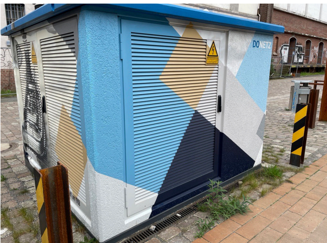
Digital local network station in Speicherstraße
