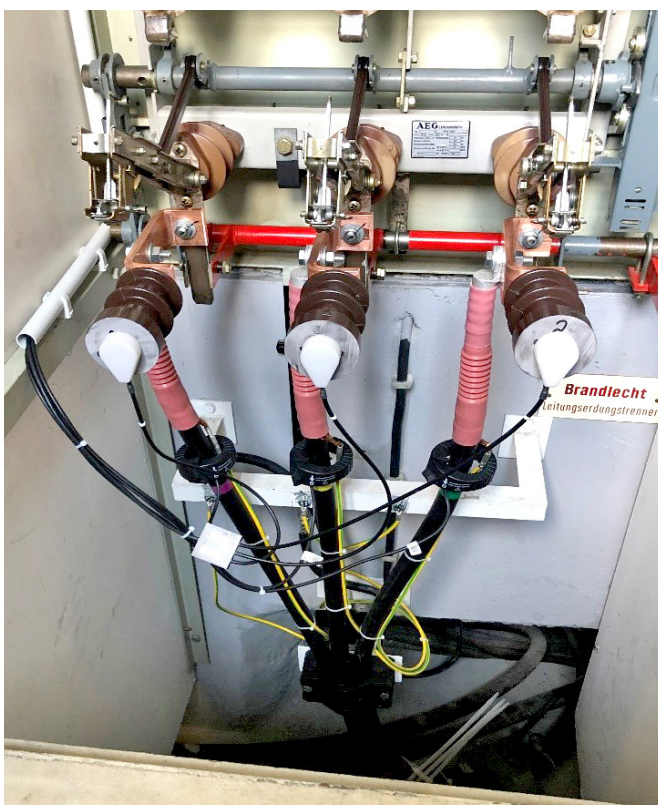
Retrofitted current and voltage sensors for load flow detection for each outgoing circuit.
