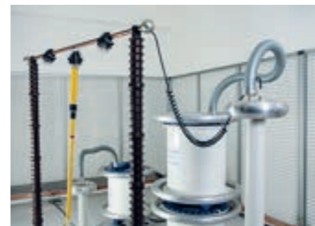
High voltage laboratory
